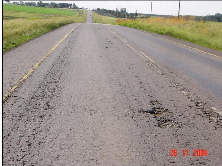
Figure 28. Surface Cracking and Potholing
