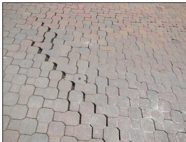
Figure 61. Excessive Openings in an Area Paved with Type S-C Blocks
