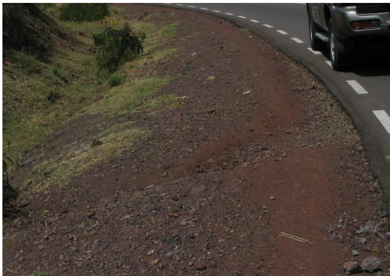
Figure 17. Unsatisfactory Unpaved Shoulder
