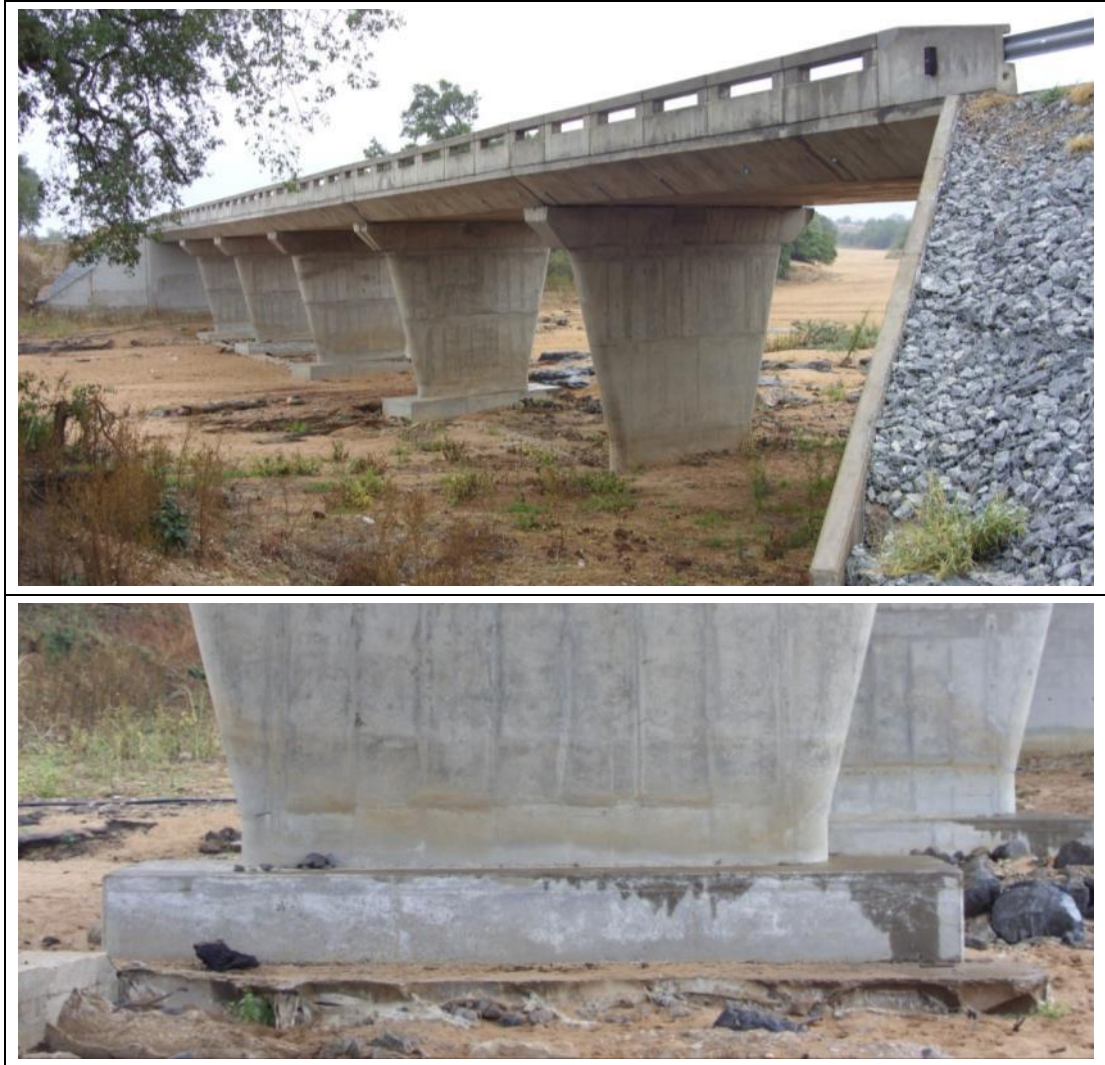
Figure 36. Scour around Bridge Piers
