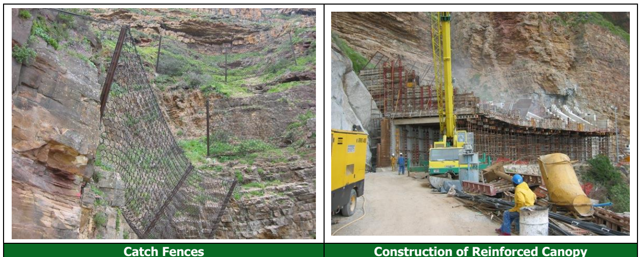
Figure 17. Catch Fences and Canopies on Chapman's Peak Drive in Cape Town
