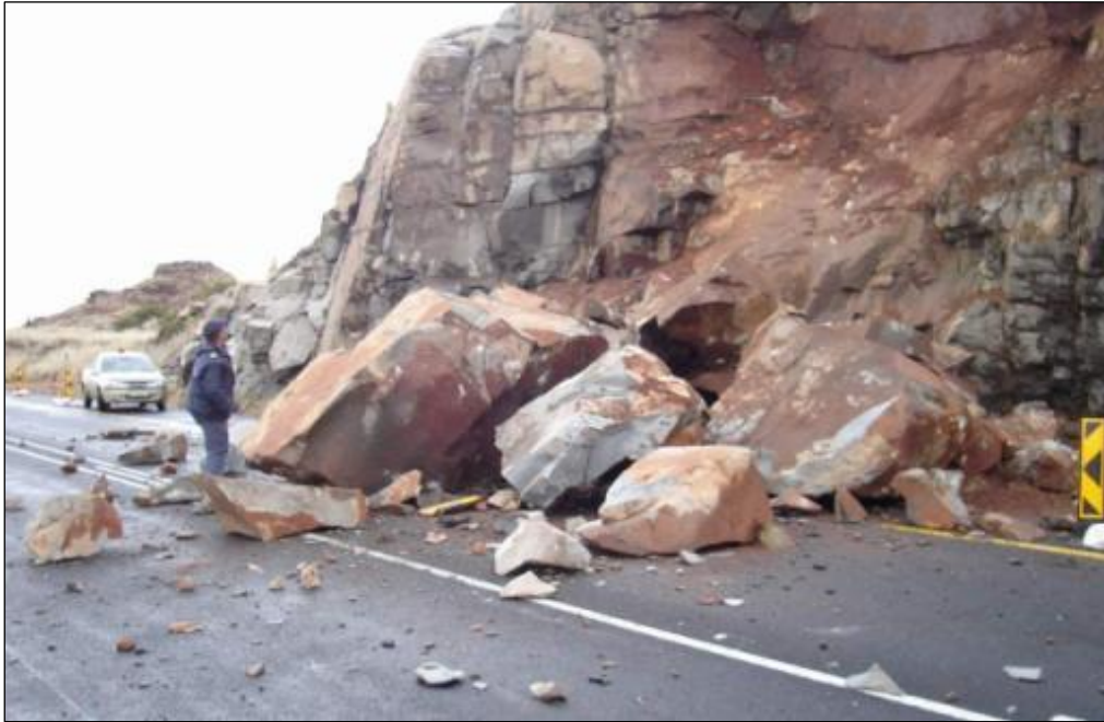
Figure 19. Toppling and Block Failures
