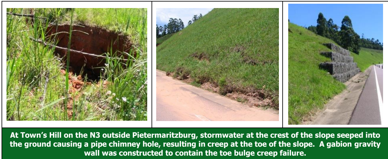
Figure 12. Internal Erosion and Piping
