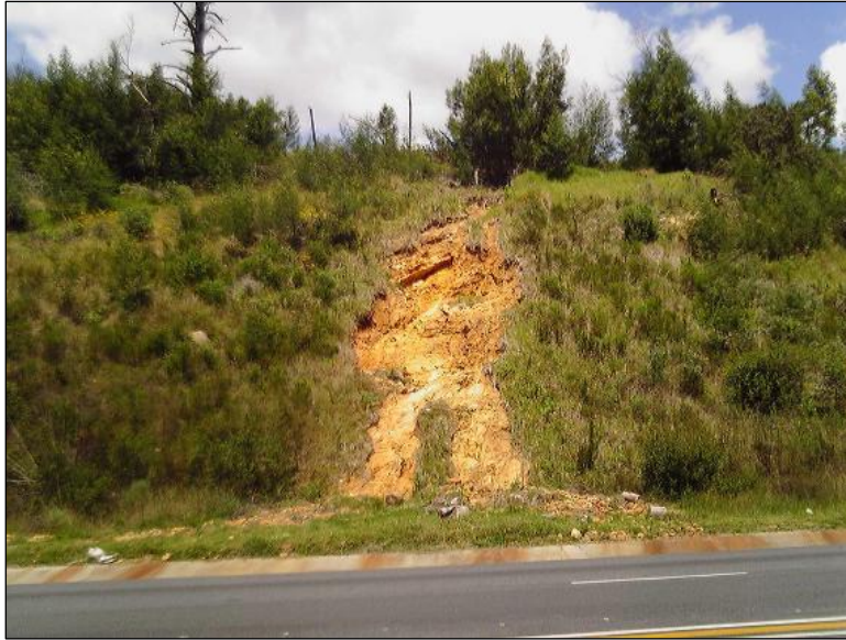
Figure 27. Erosion of Cut Face due to Inadequate Interceptor Drain above Slope
