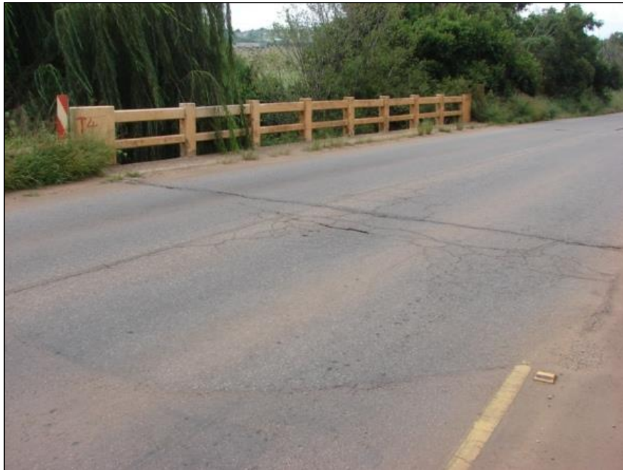
Figure 6. Bump at Bridge Approach
