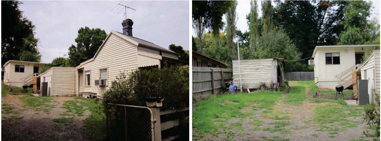
From left: east elevation showing property additions to rear and the free-standing bungalow to the rear of the property; outbuildings adjoining the east boundary.
